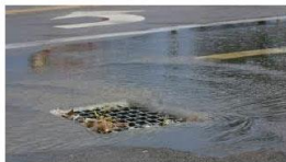
Figure 1. Drain Grate. The photo illustrates how clogged grates may pool water and increase issues related to stormwater runoff.
